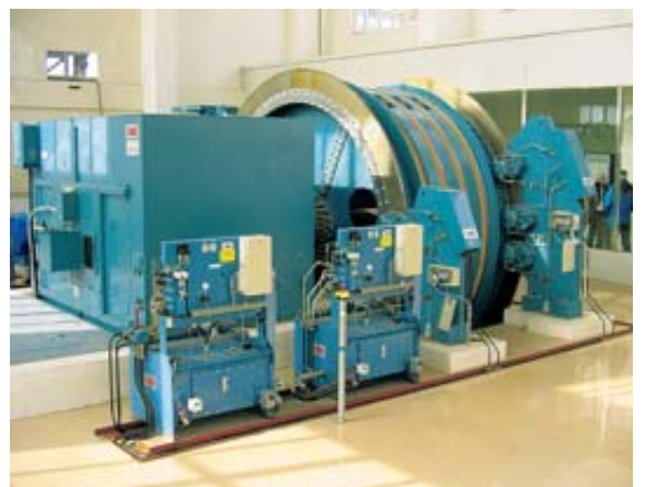
▼ Mine hoist motors
